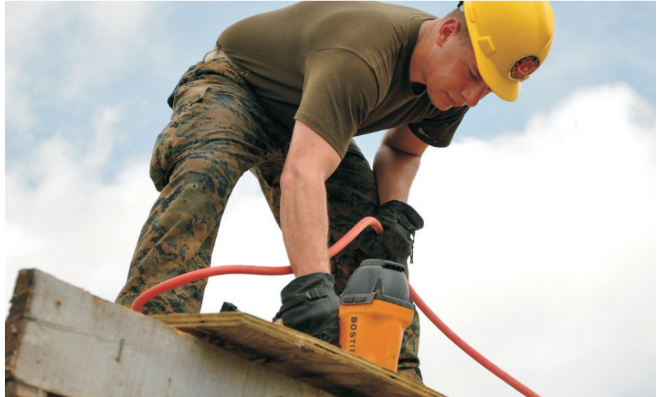
S.T.E.P.S. In The Right Direction provides housing improvement and environmental modification services as well as disaster mitigation, interior/exterior home and roof repairs, and heavy clean-up services.
